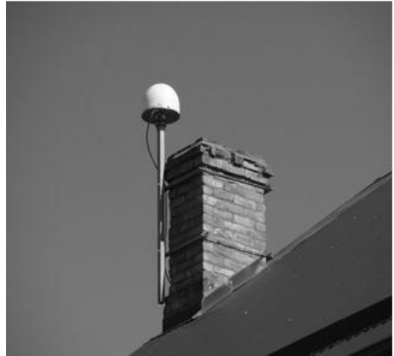
Fig.10. Base station Palsmane attachment to the chimney
